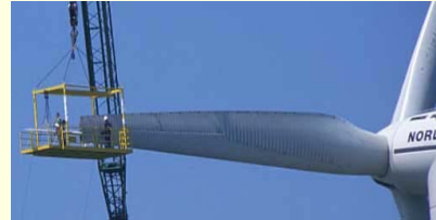
Service crew working on a 32 m rotor blade on a 1.5 MW wind turbine Photograph Christian Kjaer © 2000 DWIA
