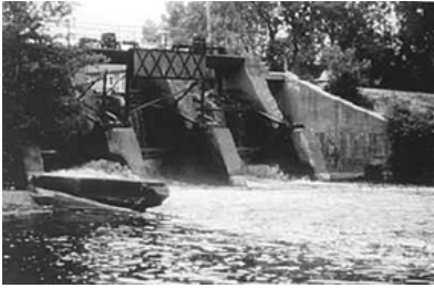
Figure 4.1 Woolen Mills Dam on the Milwaukee River before removal. Courtesy of the River Alliance of Wisconsin.
