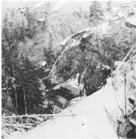
Figure S.2 Condit Dam on the White Salmon River in Washington State, a medium-size structure shown here under construction in 1913. Courtesy of Bonneville Power Authority.
